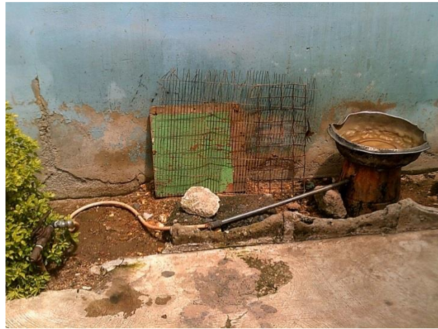
Figure 17: Bio-Digester Public Sanitation Block in Obuasi, Ashtanti, Ghana. Constructed by Impact Environmental Ltd. Biogas used to heat water for customer on specially designed stove unit.
